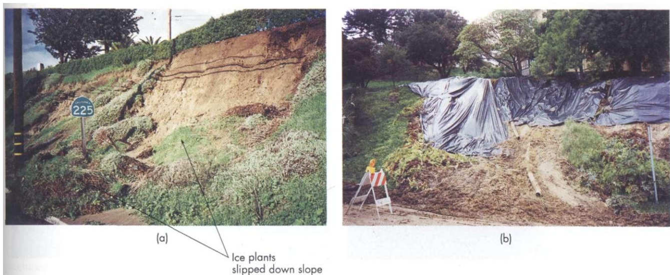
Figure 9.11 Ice plants on slopes are often unstable Shallow soil slips on steep slopes covered with shallow-rooted ice plants near Santa Barbara, California: (a) an embankment on a road; (b) a home site. The plastic sheet is an attempt to reduce infiltration of rain water. (Edward A. Keller)
